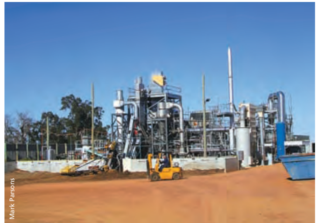
Integrated biomass fuel production plant, Narrogin, Western Australia.
